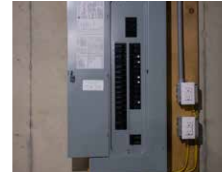
200 amp electrical service
