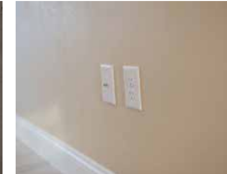
Five (5) phone & (5) cable outlets
