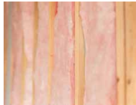
Insulation-fiberglass 5 1/2" exterior wall R21; ceiling 16" R49
