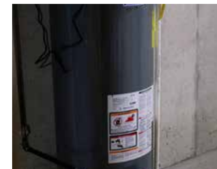
50 Gallon high efficiency hot water tank
