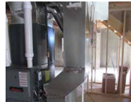
Cold air return system
